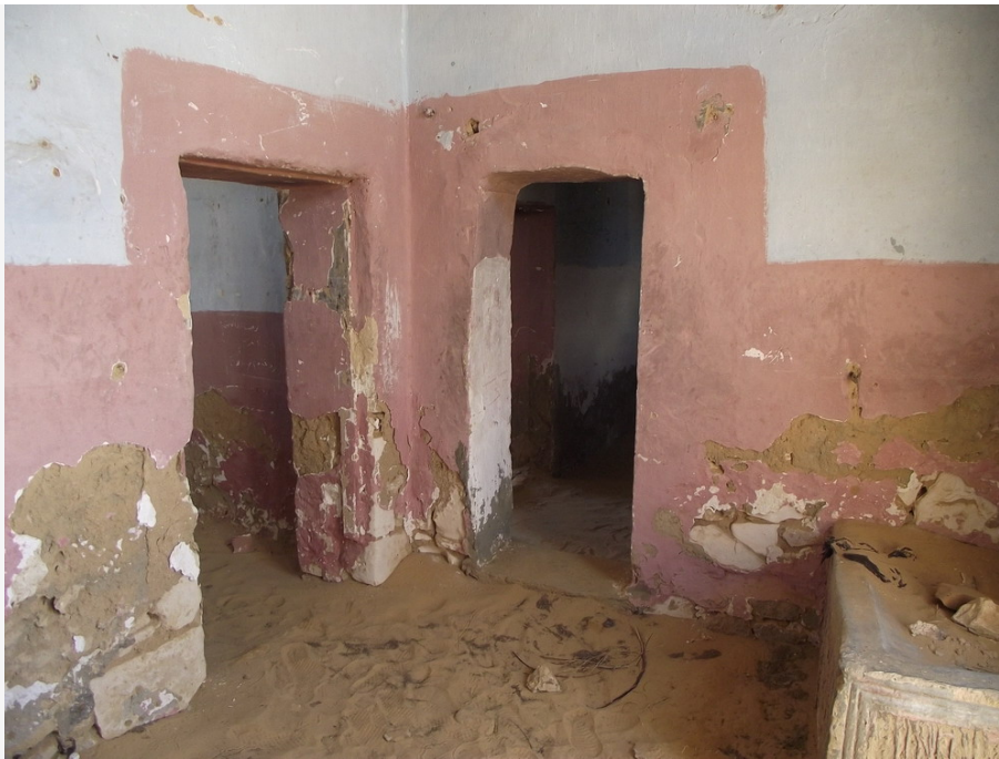
Room probably used as a reception or emergency room with different communicating entrances while all other have individual entrances.
